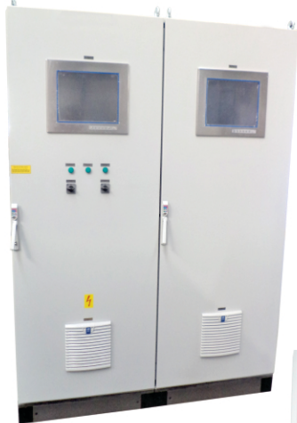
PLC Automation Panel as per customer Required
